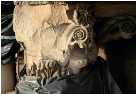
Example of a damaged capital beneath the dome.
